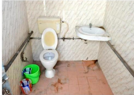
Handicapped Students Toilet - Western side
